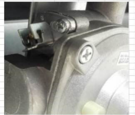
Fig. 11a: Open shut-off valve
